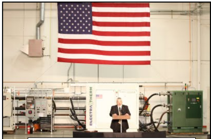
ElectraTherm's CEO John Fox spoke ahead of the President. ElectraTherm's Series 4000 machine was on display for the first time. Courtesy: ElectraTherm
