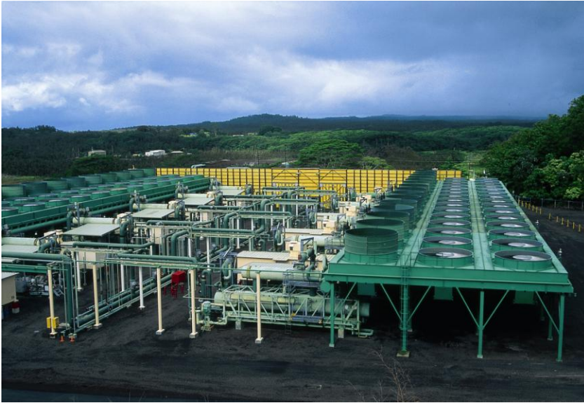
Figure 17: Puna Flash/Binary Geothermal Plant
